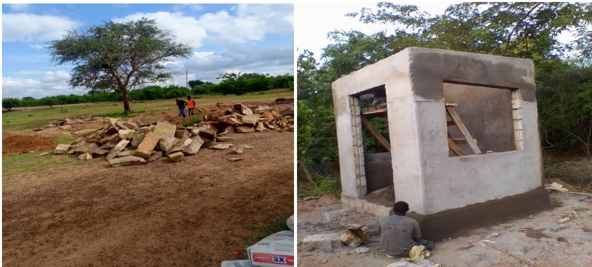
Figure 6: Photo showing the pipe line (L) and pump house (R)
