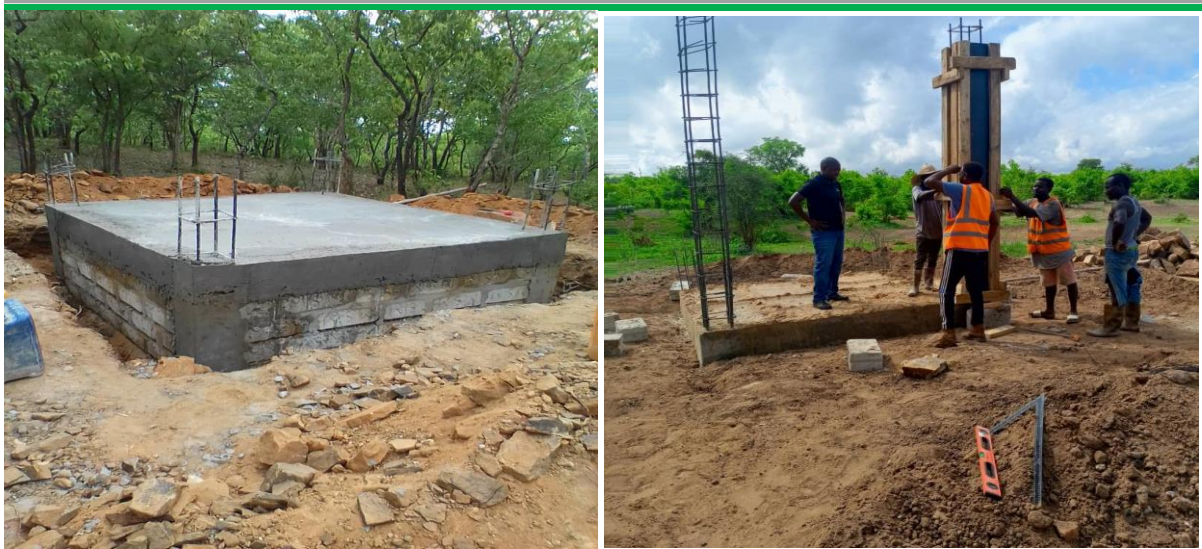
Figure 5: Photos of the foundation (L) and the tower for installation of water tank (R)
